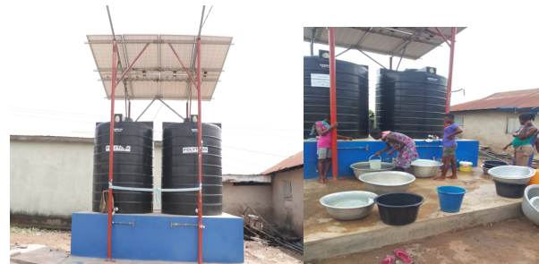
One 10,000L/Capacity Solar Water System – Pilot Project providing 3,000,000 litres of water supplied
